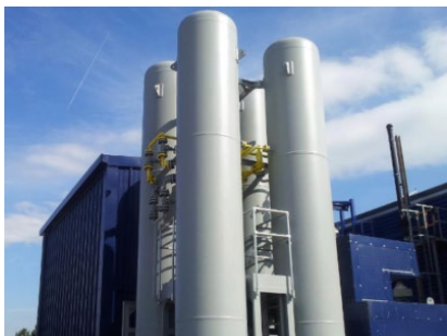
APP's Bio-SNG demonstration plant in Swindon, UK
